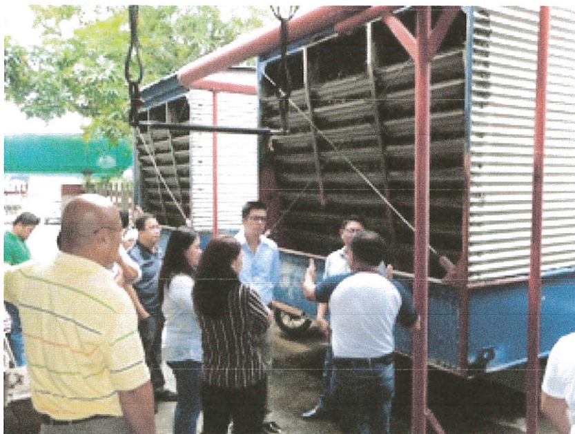
Bureau Dir. Arnold Vistan and Engr. Esteban giving the briefing during inspection of the cooling towers which are also part of the chiller system and which are to be replaced. Also in the photo are Service Chief Engr. Cliburn Cadiente and Assistant Service Chief, Engr. Jaime Galleta.
