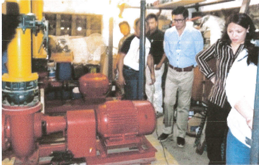
Inspection of the condenser pump room where 4 condenser pumps are located.
