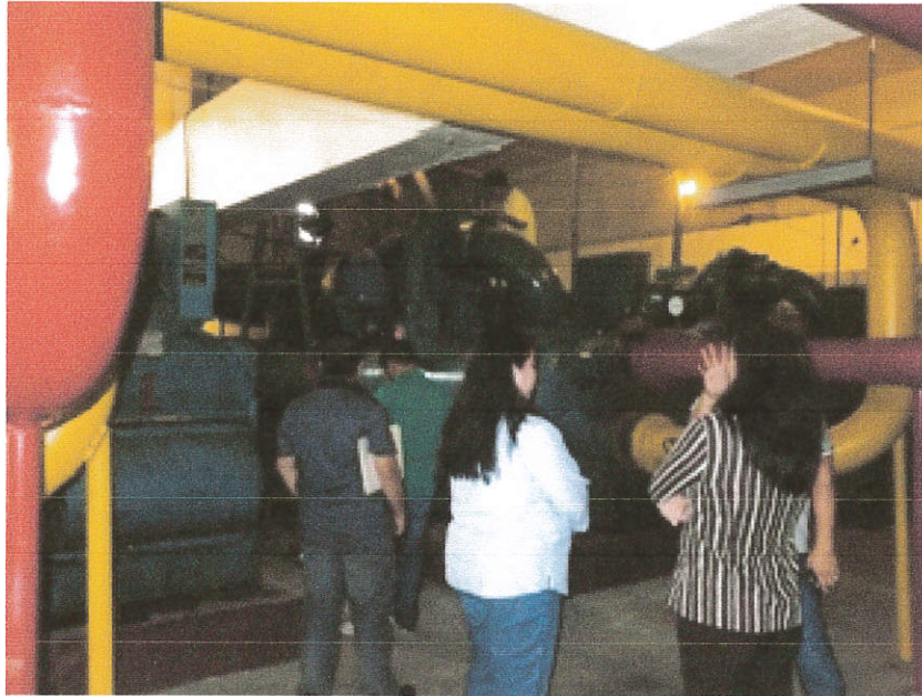
Photo showing repair and installation of existing compressor motor of chiller no. 2 as witnessed by the BAC members during the site inspection.
