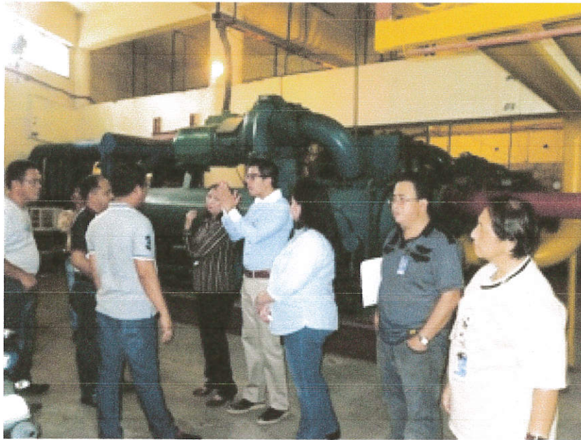
Photo showing the BAC members inquiring on the proposed location of additional 659TR chiller. Responding to queries of Atty. Bañas and Atty. Valentina Cruz (BAC Vice-Chairman) were Dir. Vistan and Engr. Esteban. Also in photo are Atty. Faye Dizon, Service Chief, Engr. Cliburn Cadiente, Rose de Castro, Head, BAC Secretariat and staff from MPFS.
