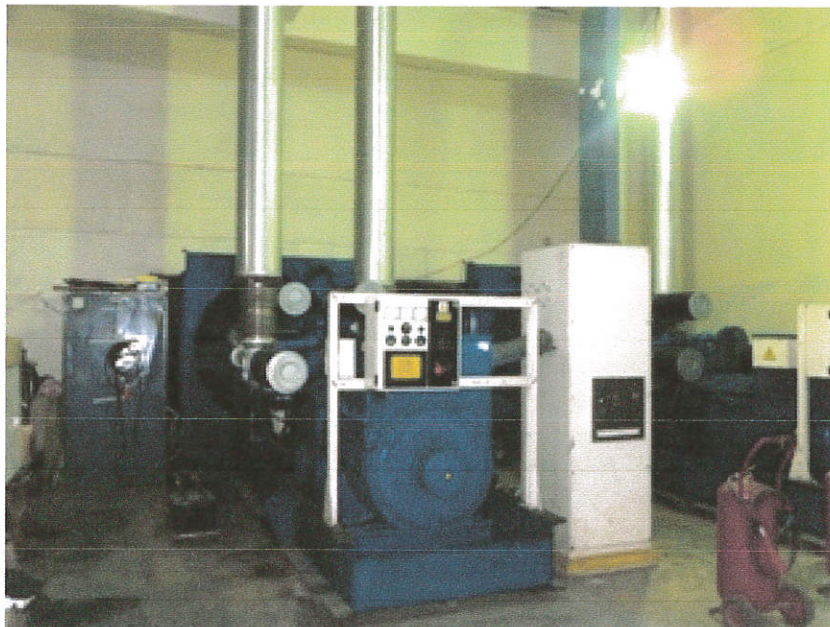
The BAC also inspected the emergency standby generator set.
