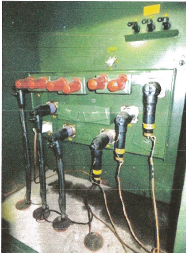
Photo showing the high voltage side of existing 2.5MVA transformer. Note the oil leaks from said unit due to normal wear and tear.
