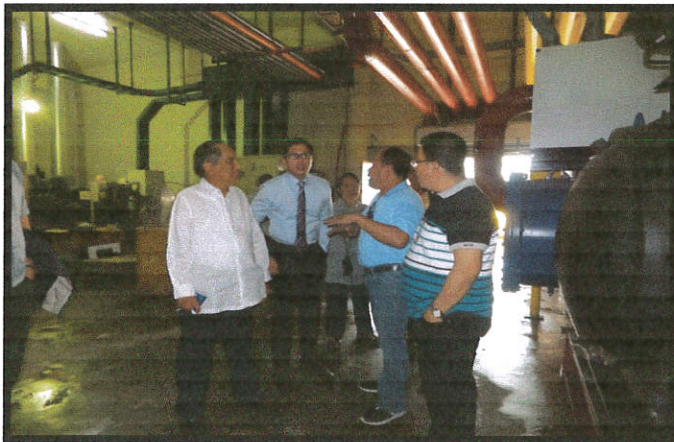
Atty. Oscar G. Yabes, Senate Secretary and BAC Chairman Atty. Arnel Jose S. Bañas inspected the site for the new chiller system with Dir. Cliburn T. Cadiente, Service Chief, MPFS. Engr. Daniel Esteban, Section Chief, Electrical Section gave a briefing regarding the said project.
